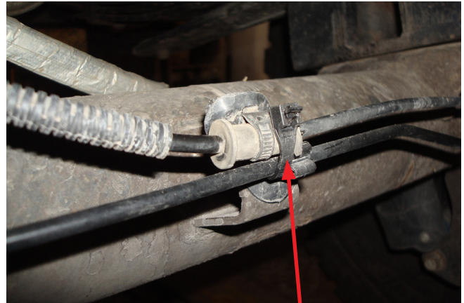
Use a zip tie and attach ABS line to brake line as shown. Fig. 11
